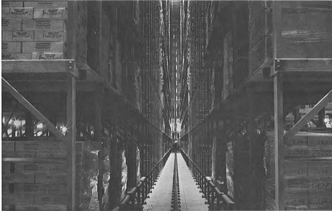
The 70-foot, computer-controlled stacker crane, shown in the background, automatically shuttles dry and refrigerated packaged products on a first-in, first-out basis at the now fully-operative Hormel plant in Austin. This automatic storage and retrieval system holds 24 million pounds of meat products.
